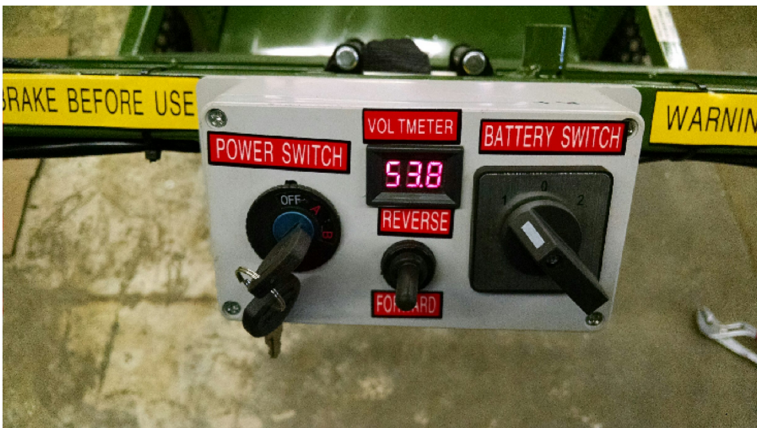
Battery Voltage Present
